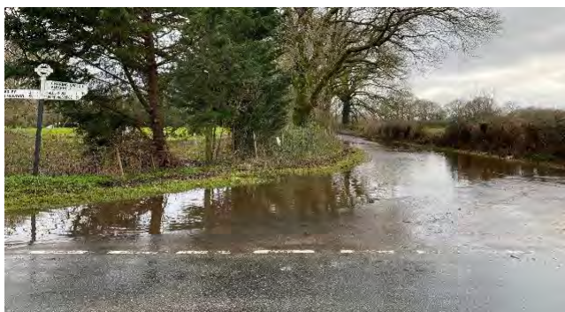
Flooding at Harbridge Drove and Drove End Junction
